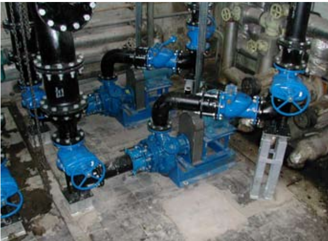
Heater recirculation plant using end suction pumps
