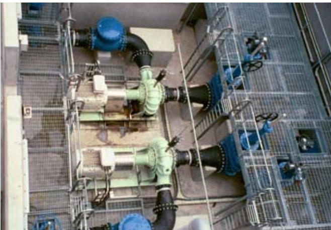
Sludge transfer station using 200 kw screw centrifugal pumps
