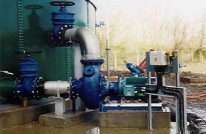
15kW - 250mm Pump Recirculating Primary Sewage Sludge on a 1000m 3 Storage Tank
